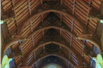
Hammerbeam roof of nave. Angels in Ceiling Beams composed of Douglas fir and Kauri
